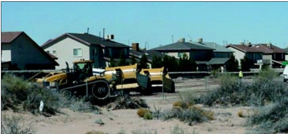
Heavy equipment knocks down scrub and levels an entrance to a new housing unit. Last year Horizon issued 341 Single Family Unit permits.
