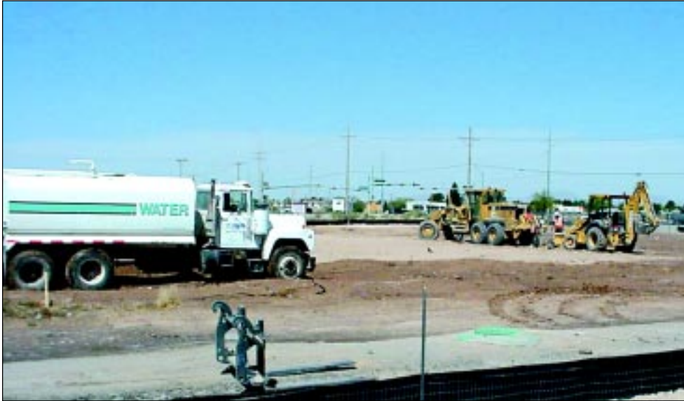
A water truck wets the ground on this property at the corner of Horizon Blvd. and Darrington so the other equipment can do dirt work. A McDonald's and Vintage Carwash will be built here. Horizon issued 30 business permits in 2007.
